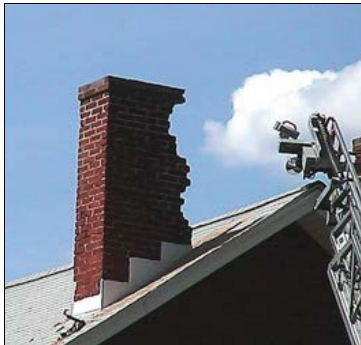
Figure 3.1.4.3.1: Chimney Damage (Fayetteville, PA) due to Aug 2011 Earthquake 49
