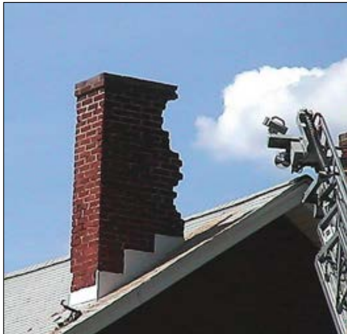
Figure 4.3.6.3.1: Chimney Damage (Fayetteville, PA) - Aug 2011 Earthquake 41
