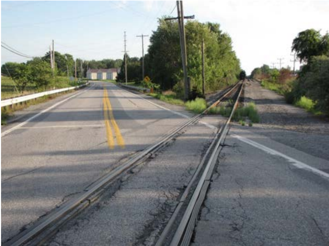
Figure 28: Unprotected Railroad Crossing of PA 433
